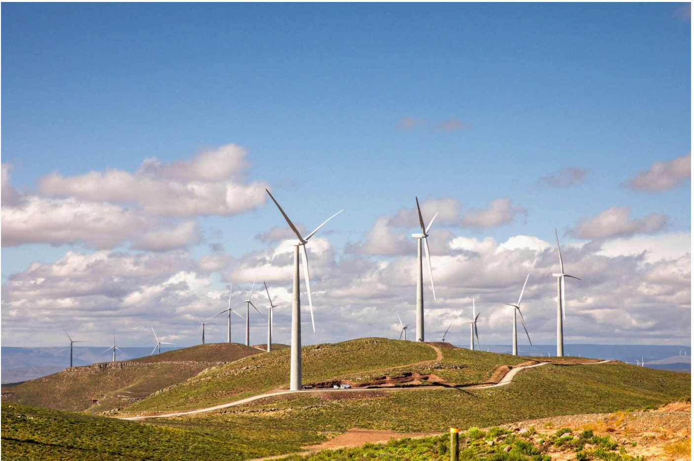
Roggeveld Wind Farm. Picture File
